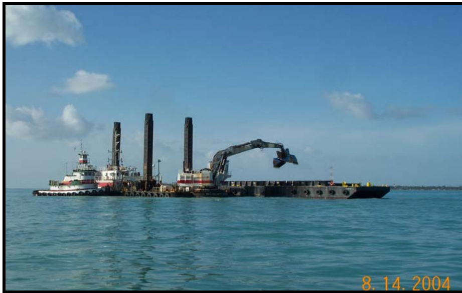
FIGURE 3.B.20. ACTIVE DREDGING BY THE NAVY CONTRACTOR OFFSHORE IN KEY WEST CHANNEL IN AUGUST 2004 (KRUER PHOTO).
